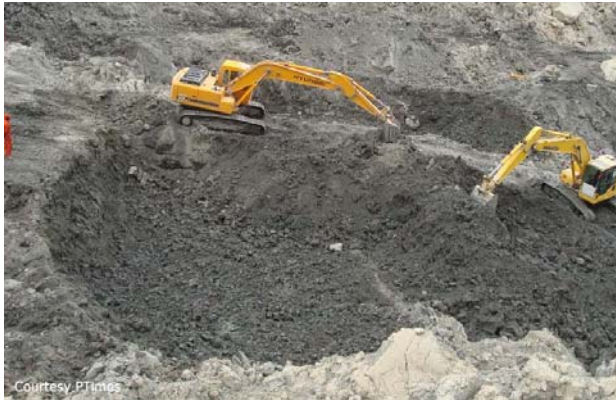
Courtesy PTimes Debris Cleaning carried out by FWO near the Lake formed at Hunza
